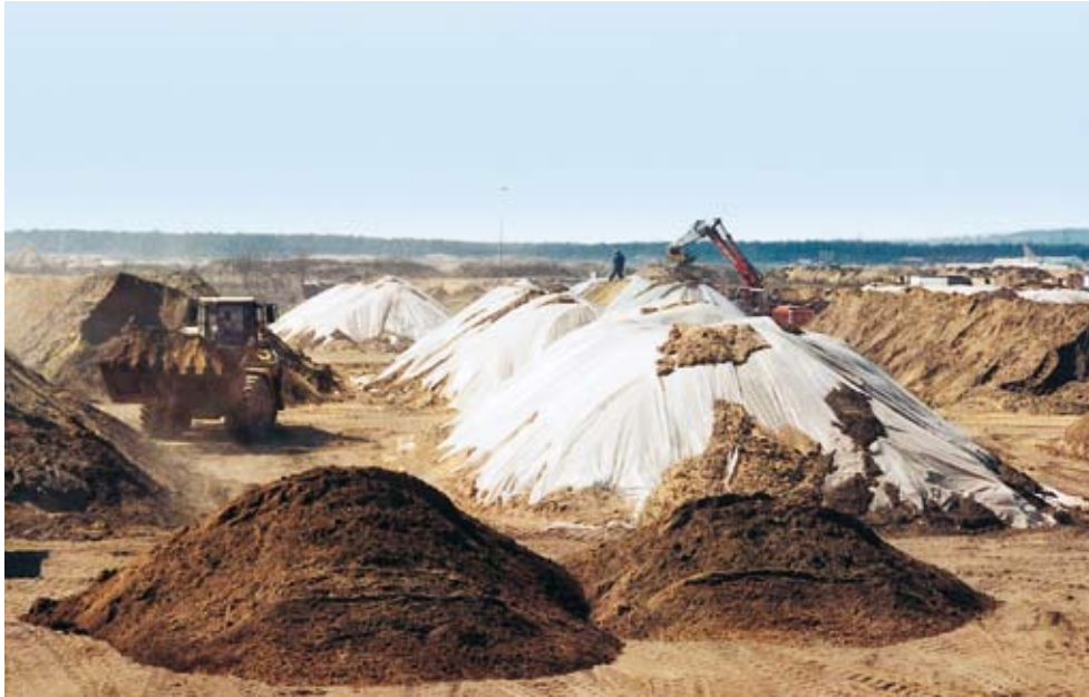
Soil and ground-water clean-up operation at Frankfurt/Main Airport: everything from one provider.
